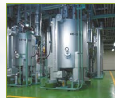
cGMP plant reactors
